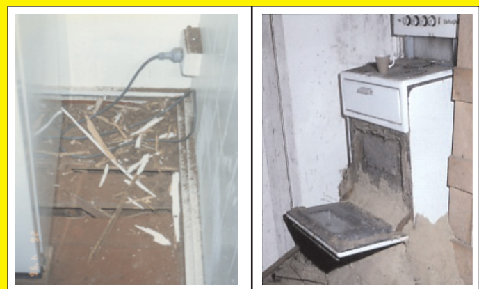
Termite damage beyond repair-don't let this happen to you.
