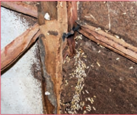
▼ Termites active in wall cavity.
