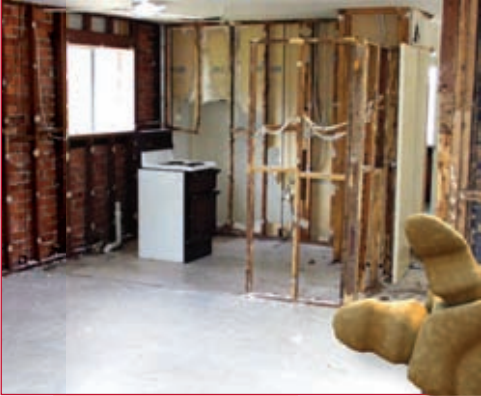
▼ $10,000 damage, not covered by insurance.
