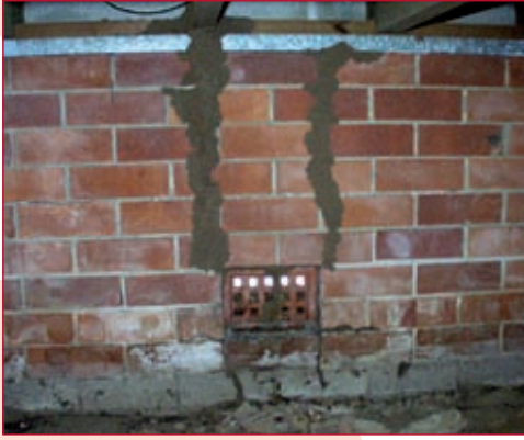
▼ Termites building mud tunnels up the brick wall and over ant capping.
